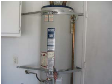
Water heater properly strapped
